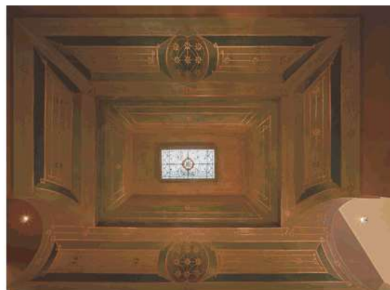
Figure 3.25 Original glass skylight and decorative hand painted ceiling above the stairs, which was uncovered by the heritage painter. Source: Images For Business, 2020.
