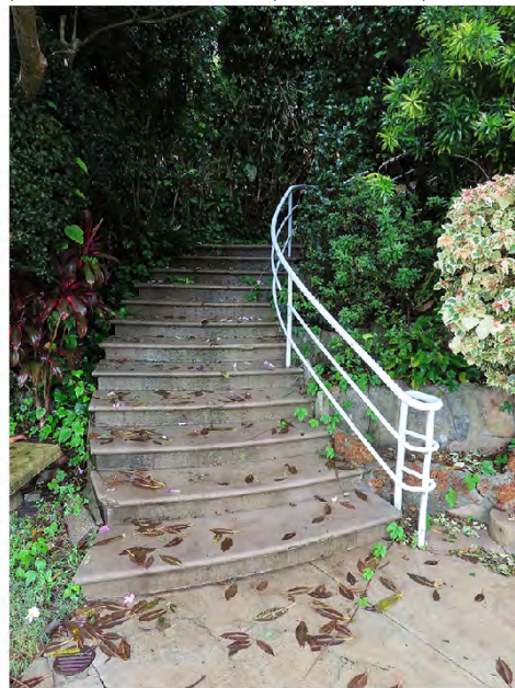
Figure 7.16: Original steps & handrail from the front garden up to the front door. (Source: Robertson & Hindmarsh Pty Ltd, 1 March 2022)
