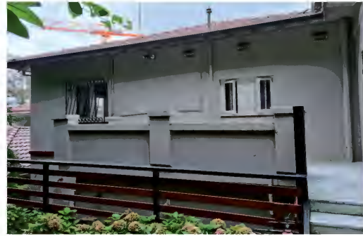
Figure 2.47 Looking to the rear (west) side of the building. Note the construction of the balcony at the rear of the building. Window frames appear to have been changed.
