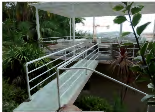
Figure 2.60 Looking to the roof terrace, showing the bridge connecting the upper level garden to the roof terrace. Note the roof terrace is covered with a steel structure and translucent glazing. The pipe railing has been replaced and the bridge was painted.
