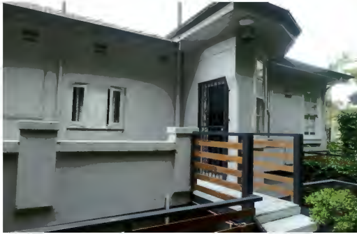
Figure 2.46 Looking to the rear (west) side of the building, showing changes to the original building.
