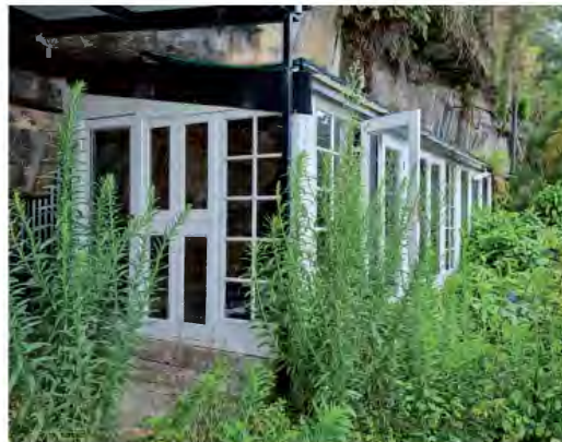
Figure 2.62 Timber structure on the north-west corner of the upper level garden, used as a gym.
