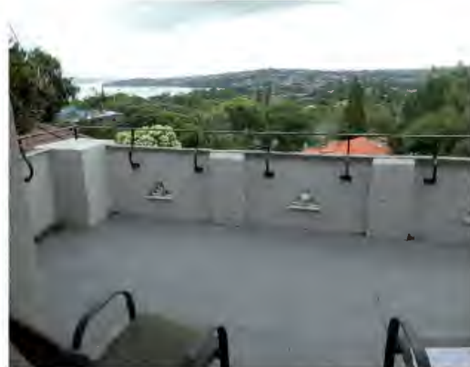
Figure 2.43 View of the upper floor balcony (originally called piazza) showing the solid decorative balustrade which was constructed later on. Note the increase the height of balustrade by the installation of steel balustrade.
