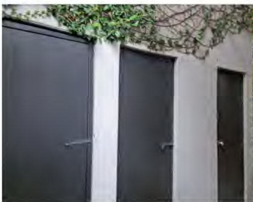
Figure 2.50 Storage area on the south-west corner of the subject site, that appears to have been constructed later on.
