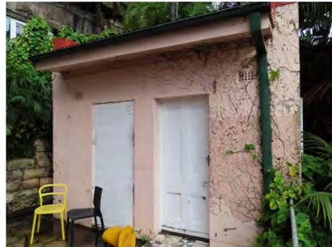
Figure 7.14: Outbuilding to the west of the house. (Source: Robertson & Hindmarsh Pty Ltd, 1 March 2022)
