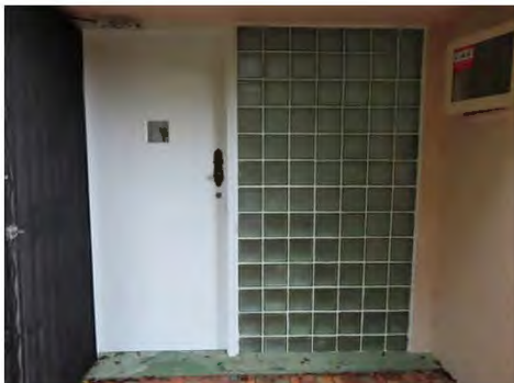
Figure 7.17: Front door with glass block sidelight. (Source: Robertson & Hindmarsh Pty Ltd, 1 March 2022)
