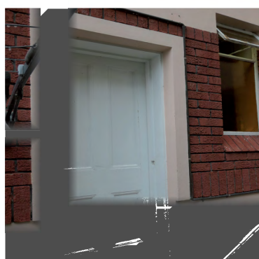
Figure 2.56 A new timber door to the front garden for the bedroom on the basement.
