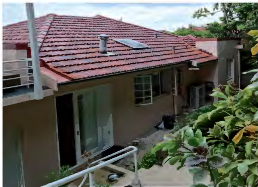
Figure 2.59 Looking to the rear (west side) of the building, showing changes to the original openings, and the installation of skylight on the roof.
