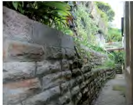
Figure 2.64 Looking to the rear (west) side of the house, showing the stone wall and bridge.
