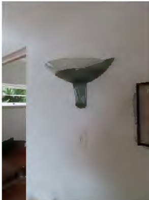
Figure 7.21: Entry wall light and original light switch plate beneath. (Source: Robertson & Hindmarsh Pty Ltd, 1 March 2022)
