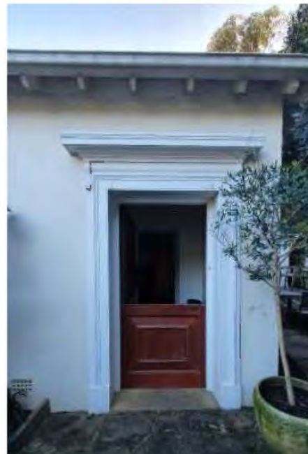
Figure 13 View of the front door with entablature. This details matches the State Library drawings.
